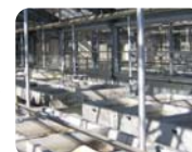
Water tanks in the conservatory
